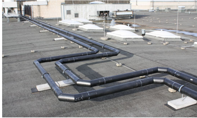
Fig. 7.3.1. Built in lyre to withstand stress in the pipe system. [1]
